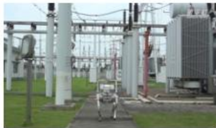
Jinan Substation Intelligent inspection
