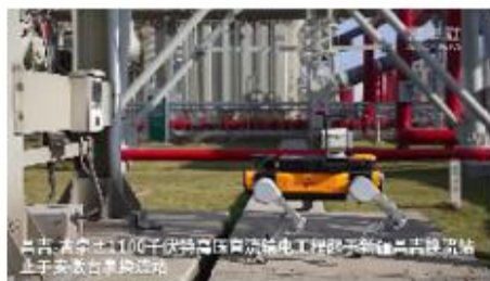
Anhui Guquan Converter Station Inspection
